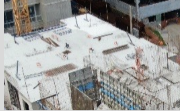
Non-existent or incomplete guardrail
