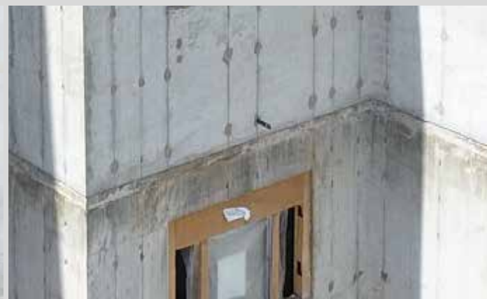
Lack of façette removal
