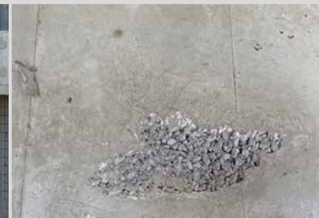
Segregation of concrete
